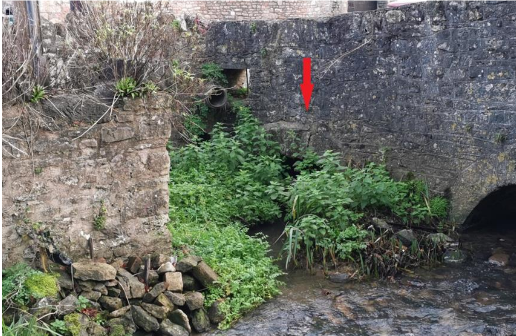
Figure 14 - Jack's Bridge showing the culvert adjacent to A371 Long Street blocked with vegetation
