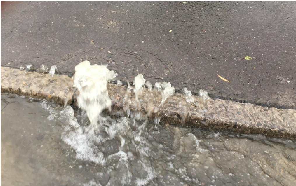
Figure 17 - Cracks in Long Street from which water was reported to be emanating.
