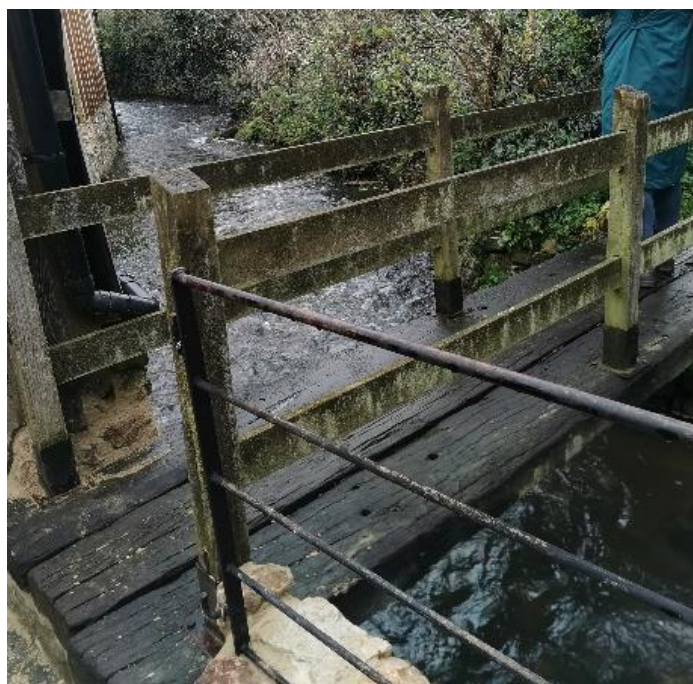
Figure 13 - Example of private bridge to the rear of properties on A371 Long Street
